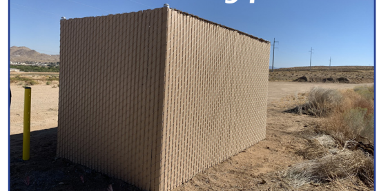
The upper pond PLC has a new look with a desert toned fence. The PLC operates valves used to feed recycled water to the upper percolation ponds.
