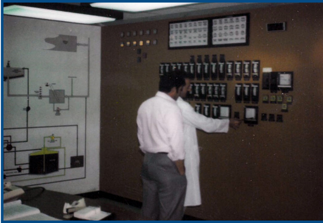
SCADA at VVWRA in the 1980's.
