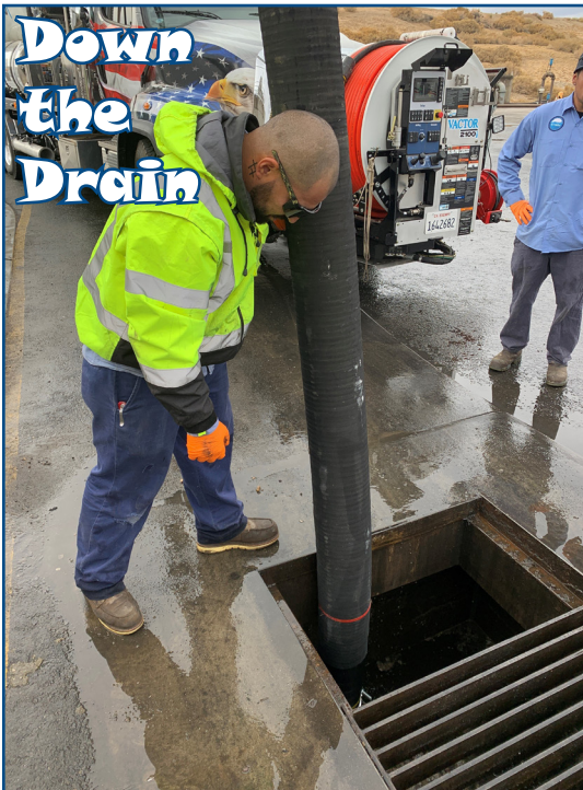
Maintenance Mechanic-in-training Juan Alvarez uses a vactor truck to clean out a drain following a recent storm.
