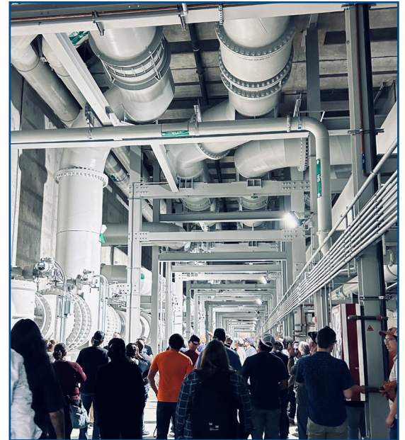
CWEA members get a look at the massive underground gallery of piping at Echo Water.
