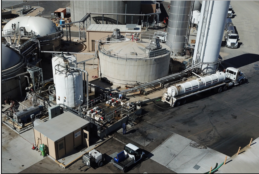
An aerial view of the ADM receiving area where food waste is delivered.
