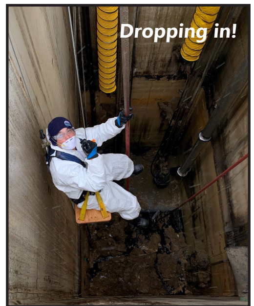
Mechanic-in-Training Allen Dorado is lowered into a wet well in Hesperia to help remove rags, wipes and other debris.
