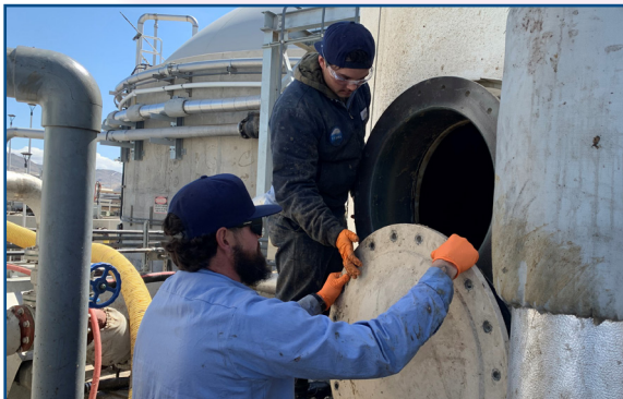
Mechanic James Carothers lifts an ADM tank cover as Mechanic in Training Allen Dorado helps set the lid in place. ADM is food waste that generates methane that is converted into renewable natural gas.
