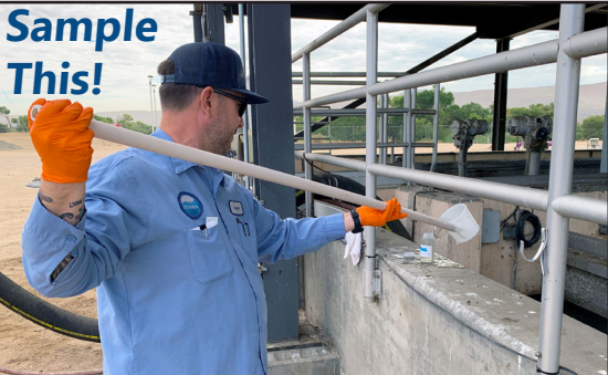
Operator-in-training James Pasieka taking a sample of recycled water at the tertiary filters.
