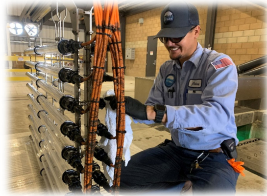
Inside the UV Building at the Regional Plant
