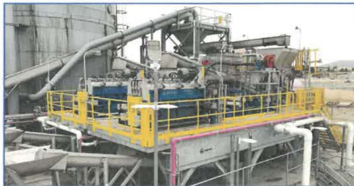
An organics polishing system similar to this one will be installed at VVWRA.
