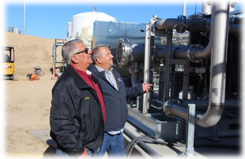
Renewable Gas Project at Victorville Plant
