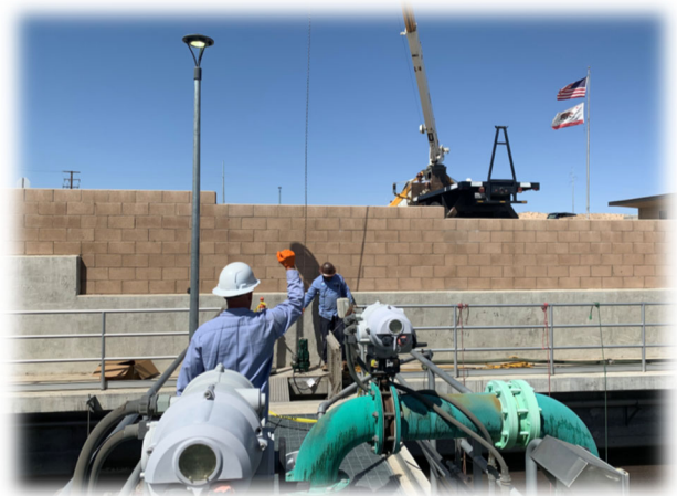
Hesperia Sub-Regional Plant
