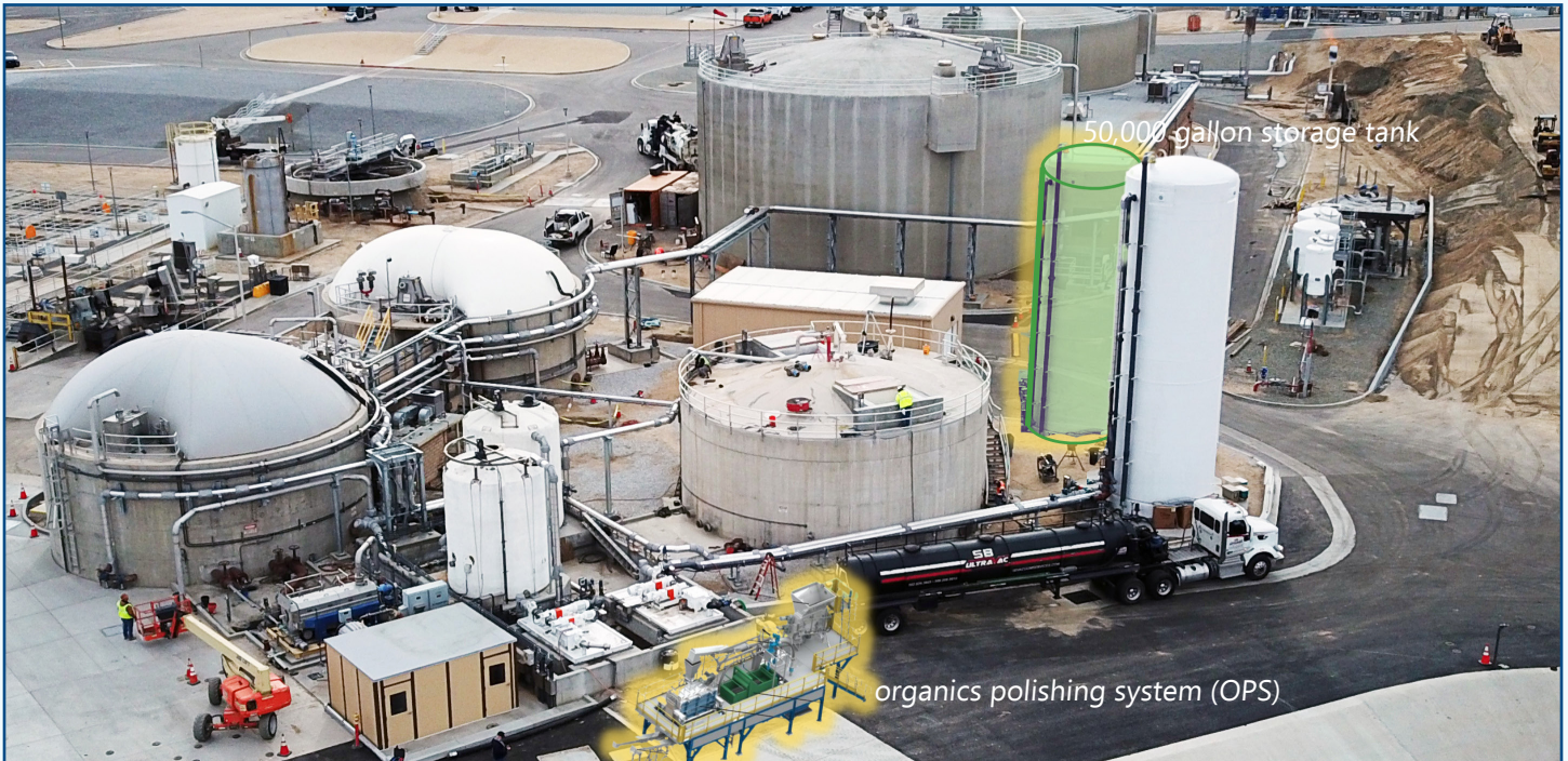
Artists rendering of where the new organics polishing system and storage tank will be located at the ADM delivery area.
