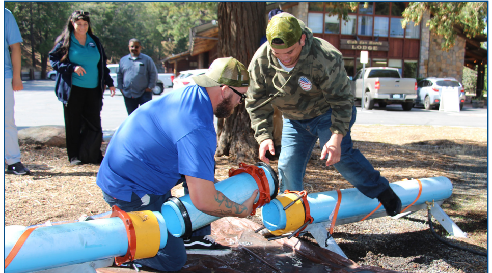
Lead Operator Kalin Westover (l) and Operator Moises Castro compete in a pipe repair competition at the DAMS Vendor Fair and Training at San Moritz Lodge in Crestline.
