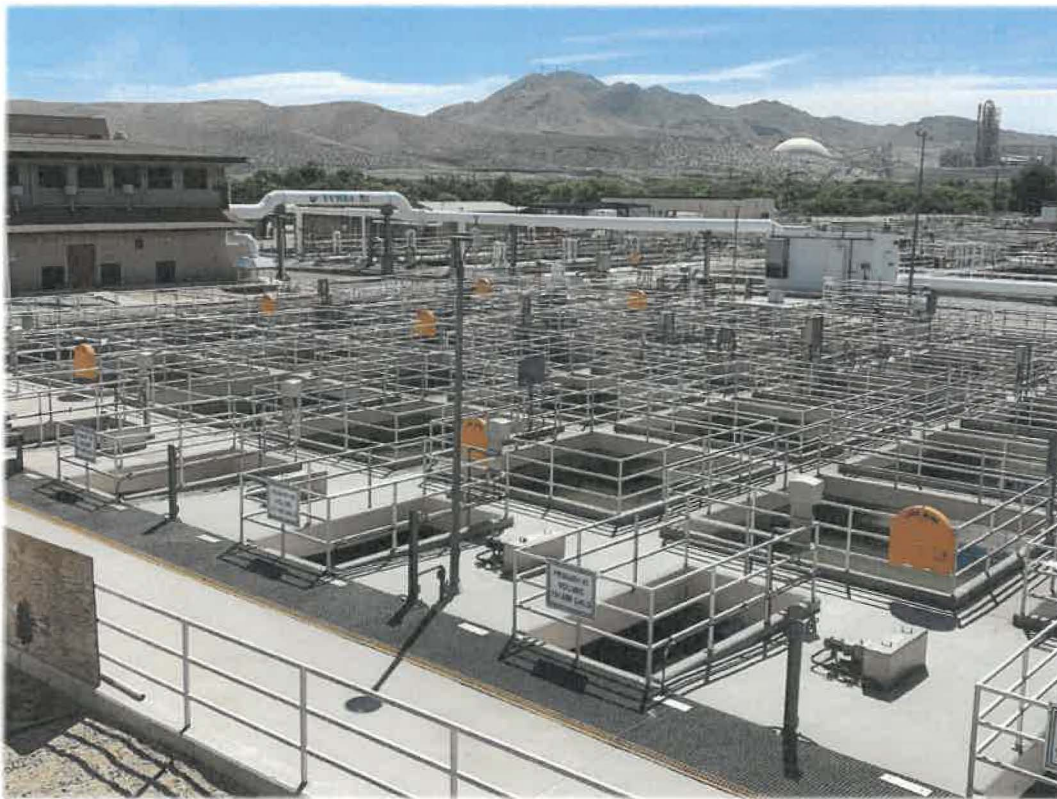
VWRA Regional Plant
