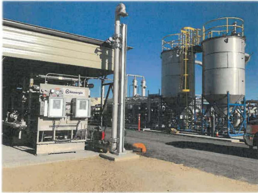
Renewable Natural Gas Project
