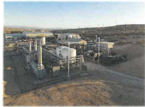
Regional Plant Renewable Natural Gas Project
