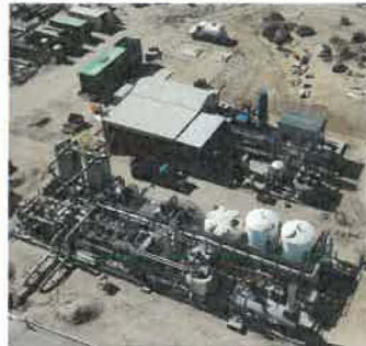
Gas is scrubbed and pressurized to become RNG.
