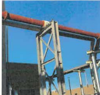
Pipeline transports biogas.
