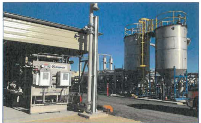
The RNG conditioning facility where methane or biogas is converted into renewable natural gas.
