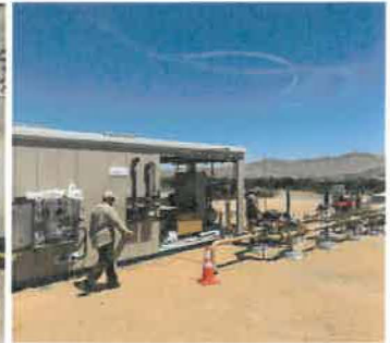
RNG is injected into a Southwest Gas pipeline.
