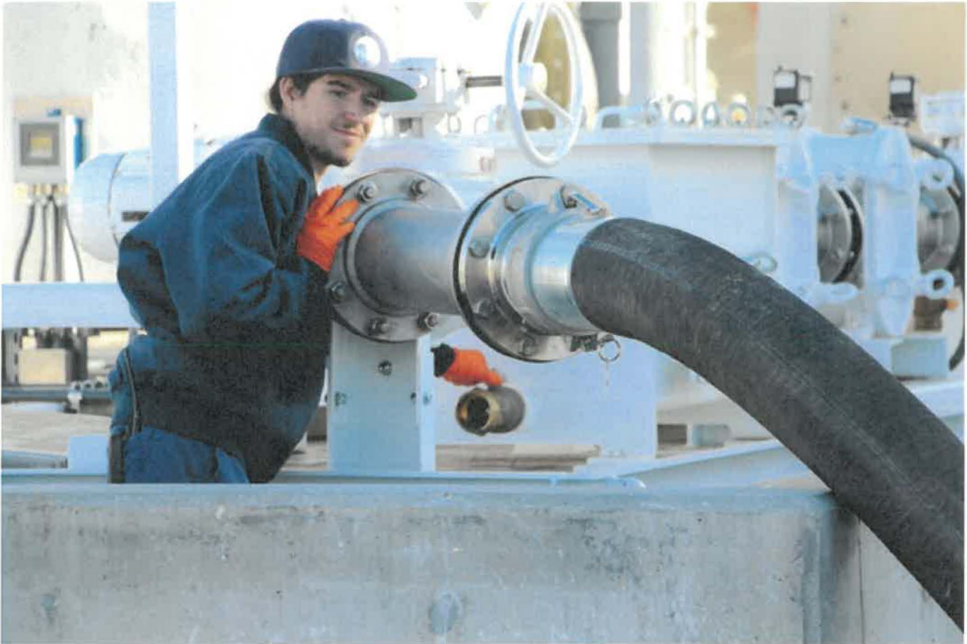
VWRA's Brandon Talley watches as the first load of food waste is pumped into the digesters.
