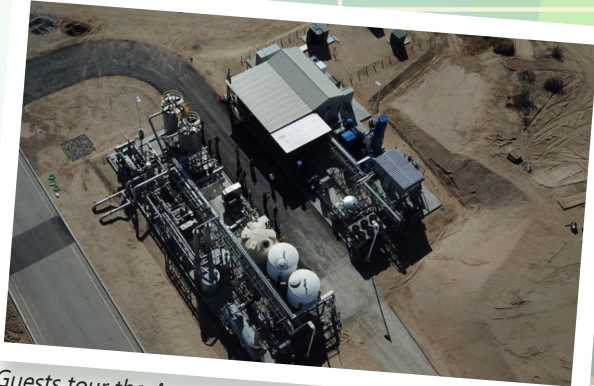
Guests tour the Anaergia gas conditioning facility.
