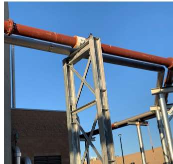
Pipeline transports biogas.
