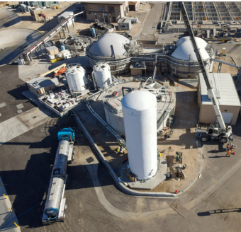
Truck delivers food waste to digesters.
