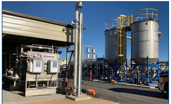
The RNG conditioning facility where methane or biogas is converted into renewable natural gas.
