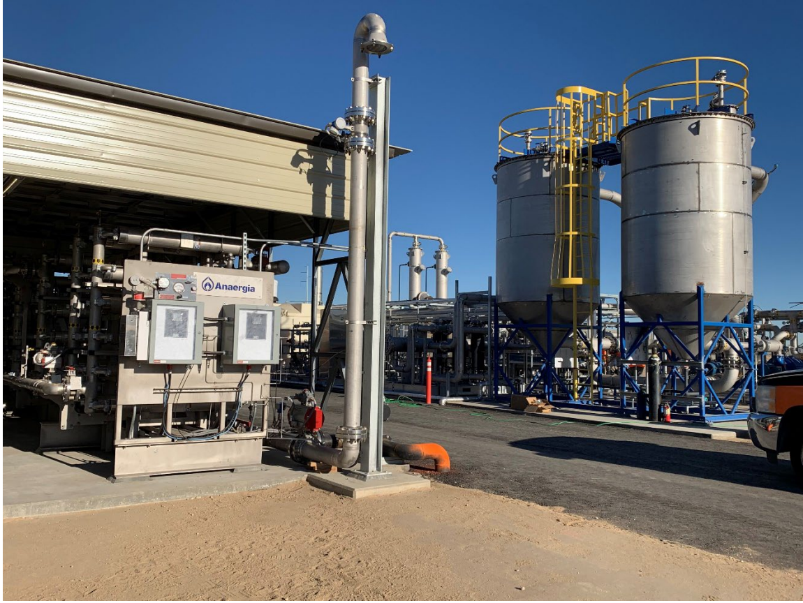
Biogas treatment facility where methane or biogas is scrubbed (cleaned) and converted to RNG.
