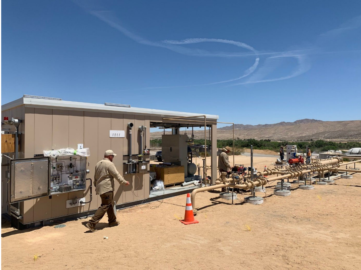
This is the site where cleaned and pressurized RNG is injected into a Southwest Gas pipeline.
