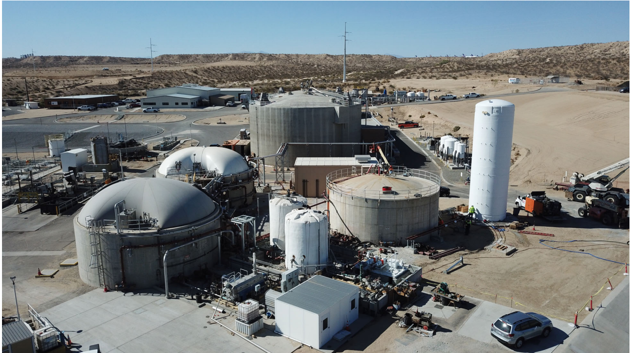
Renewable Gas Project at Victorville Plant
