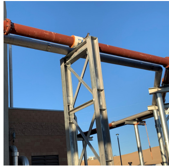
Pipeline transports biogas.
