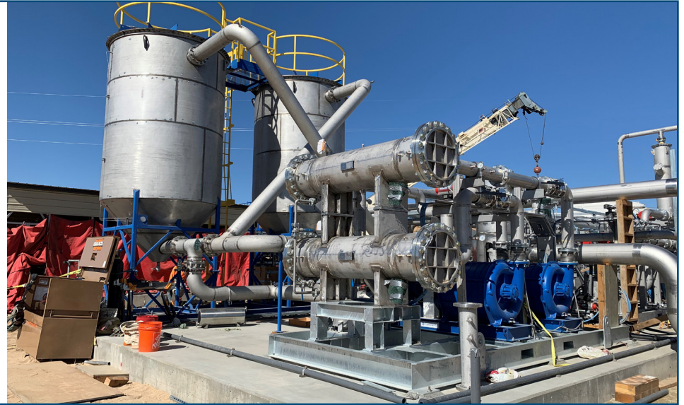
A gas scrubbing facility which cleans and pressurizes biogas to bring it to RNG standards.
