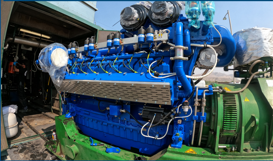
One of two MWM 800 kwh generators recently installed at VWRA.
