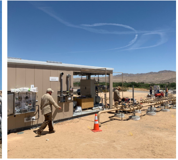
RNG is injected into a Southwest Gas pipeline.
