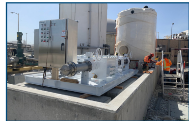
New food waste receiving station.
