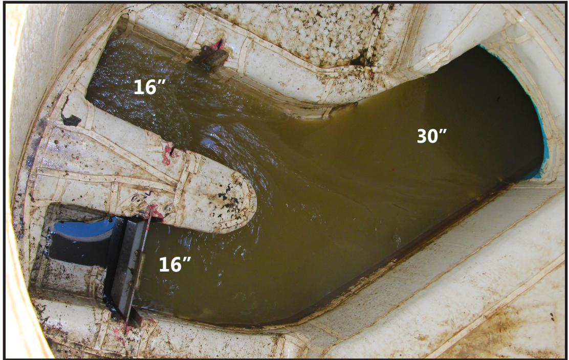
Wastewater flowing from a 30" pipe to two new 16" pipes that go under the Mojave River and join the large pipeline drilled through a rocky hillside in the Upper Narrows.
