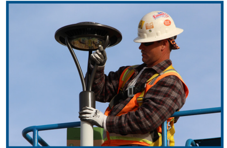
New 78 watt dome hat LED light installed by Aaron Rister from Big Sky Electric
