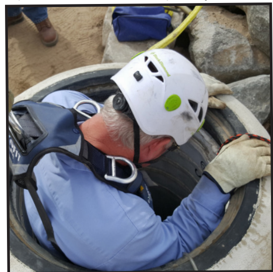
VVWRA's Robert Townsend enters a manhole to pull the plug that opened the newly finished Apple Valley sewer lines.
