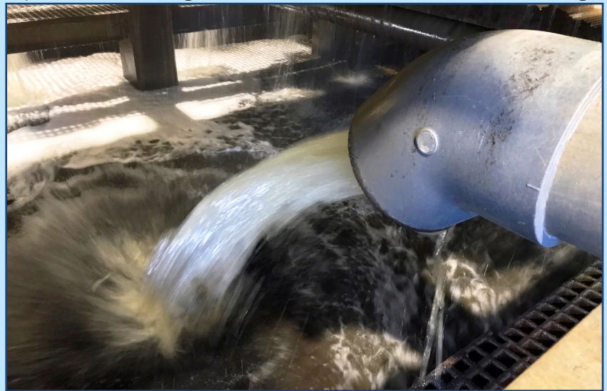
Water separated from sludge in the GBT is returned to the plant for treatment.
