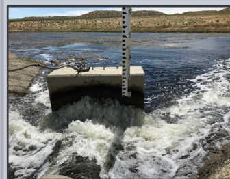
Recycled water flowing into perc pond 8.
