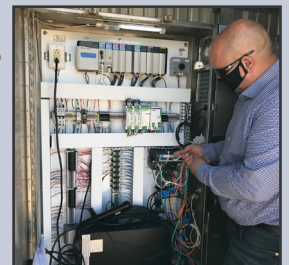
PLC at perc pond 8.
