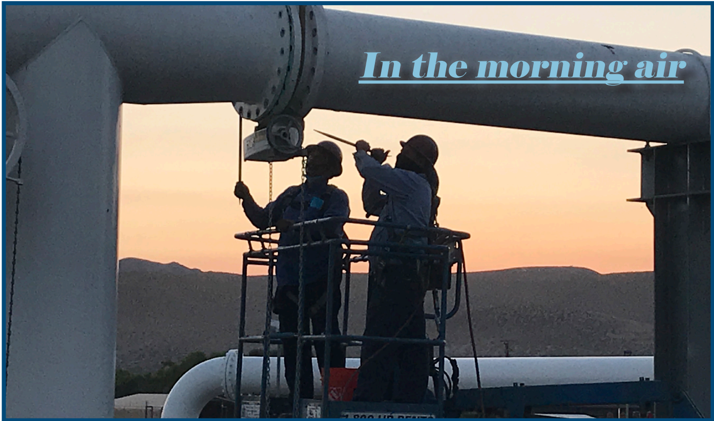
Maintenance Mechanics Marcos Avila (l) and Richard Swatzell (r) work on replacing a valve on the air header in the early morning hours. They were on a lift about 12' off the ground. The large pipe carries pressurized air to our aeration basins which provide oxygen to sludge eating microbes.
