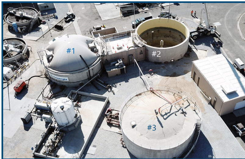
Aerial view of the 3 original digesters that are being rehabbed at VVWRA.
