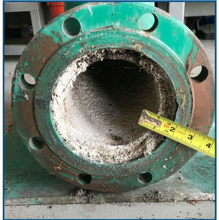
Struvite found inside a pump cavity.
