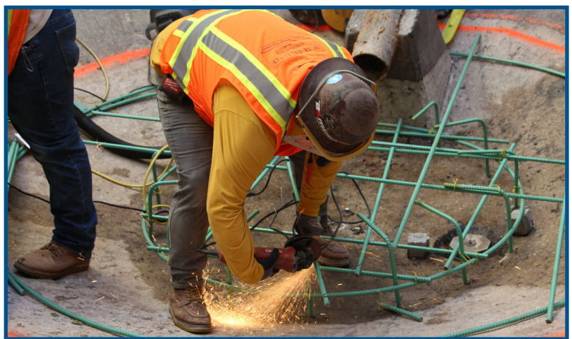
A worker with W.M. Lyles cuts rebar at the bottom of digester #2.
