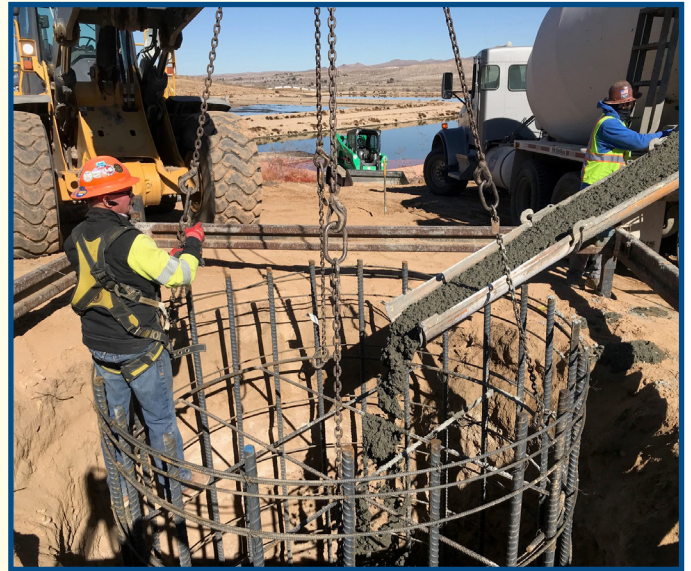
A base hole 32 feet deep and ten feet wide was filled with 100 yards of concrete.
