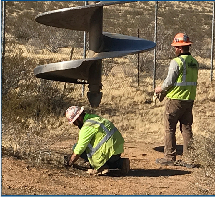
Workers prepare the site and move a large auger into place before beginning to dig.
