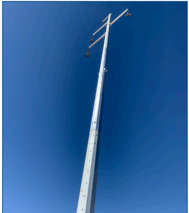
Fully assembled power pole. Power lines will be installed with the help of a helicopter.
