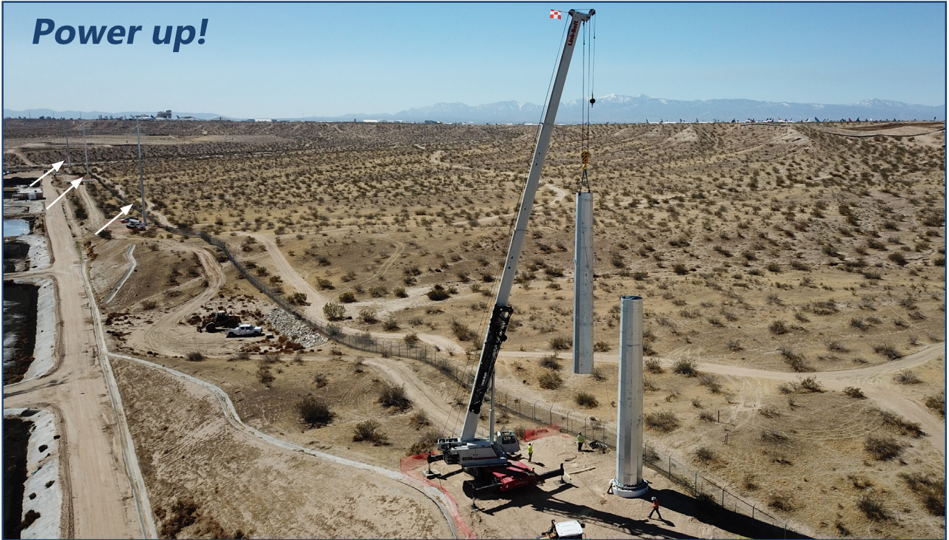
Workers use a crane to put in place the second section of a three-piece power pole along VWRA's western fence line. It is one of four new high voltage power lines installed on VWRA's main plant. The arrows indicate their locations. Two more poles are being installed further to the south adjacent to our south percolation ponds.
