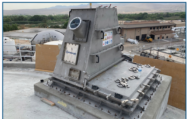
One of 3 new service boxes on top of digester #4.
