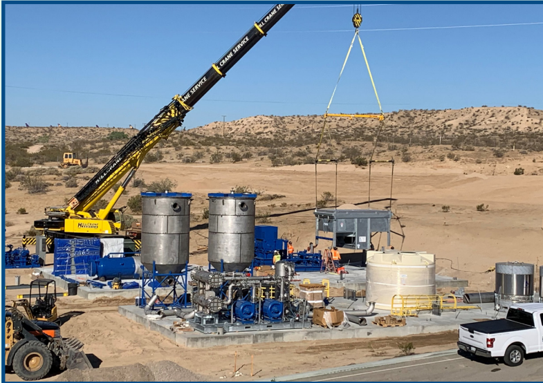
Aerial view of the gas scrubbing facility.
