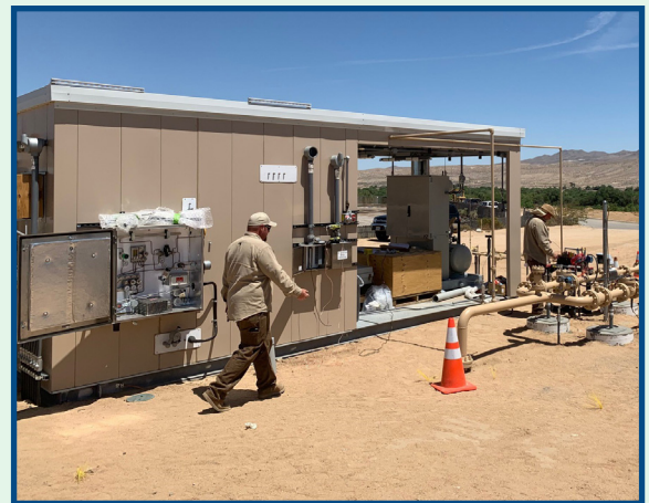
SWG gas injection site.
