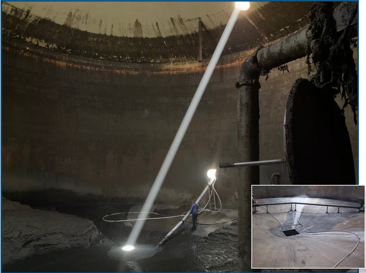
A beam of sunlight through a port opening creates a dramatic scene as Maintenance Mechanic Marcos Avila uses a steel extension attachment from a vactor truck to vacuum out a large amount of grit and sand at the bottom of Digester #4. Clean digester floor (inset photo).
