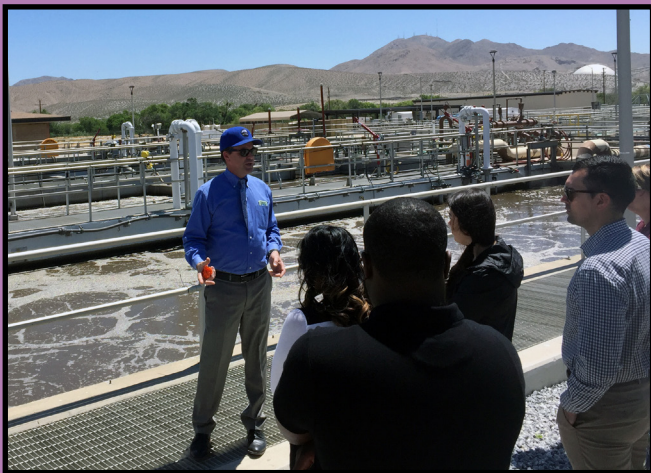
VVWRA GM Logan Olds explains the aeration process to Leadership group.
