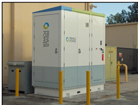
Primus Power battery storage at another facility.
