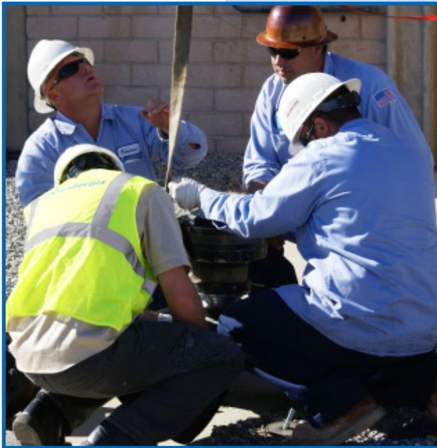
VVWRA's Mike Koncur, Richard Swatzell and Brad Doneff work with a contractor on a mixing mechanism taken from inside the Omnivore digester.
