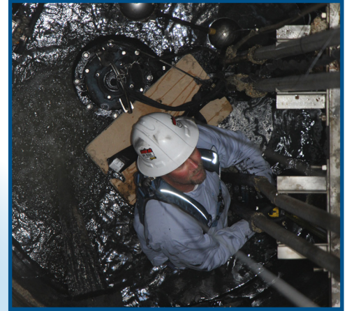
Mechanic Brian Fenton makes repairs to a pipeline inside a 40 foot wet well.
