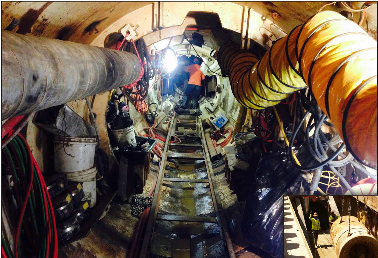
A view inside the 84" Upper Narrows tunnel where it meets a smaller 60" tunnel underneath C St. in Victorville. Large pipes will fill these tunnels to carry wastewater from the east side of the Victor Valley back to VWRA.
