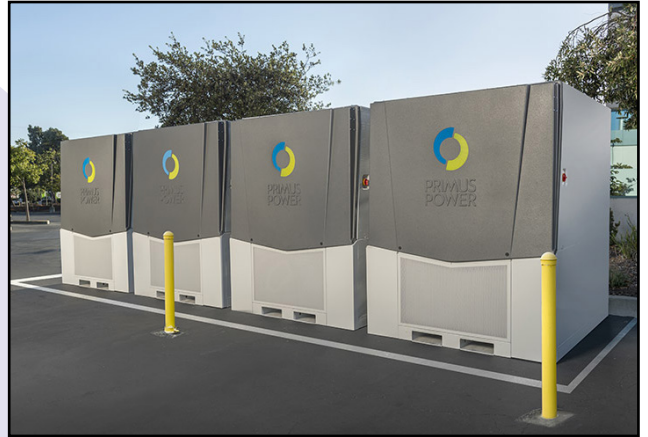
VWRA is installing eight Primus Power flow cell batteries similar to these. The batteries will store power that can be used during power outages and maintenance.
