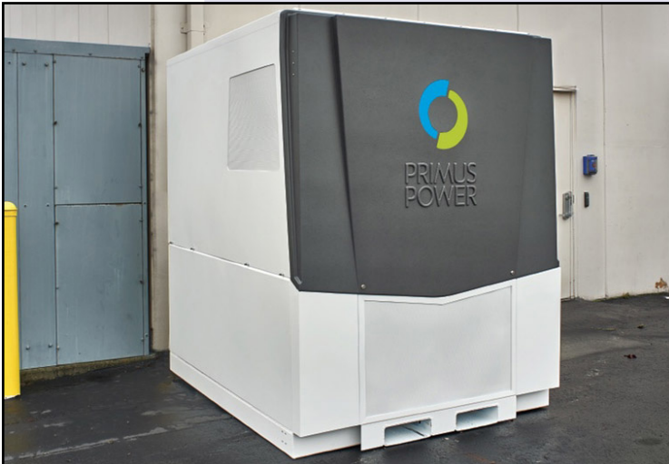
Another look at the Primus Power zinc bromide flow cell battery with titanium electrodes.
