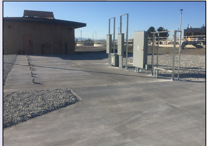
A new concrete slab has been poured at the site where the batteries will be installed. The site will include outdoor lighting and the microgrid will be located inside the existing building.
