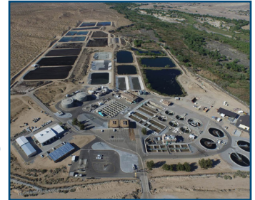
Aerial view of VVWRA.
