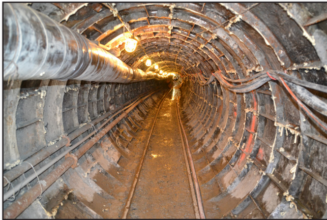
This picture was taken about 300' inside the tunnel being drilled at the Upper Narrows
