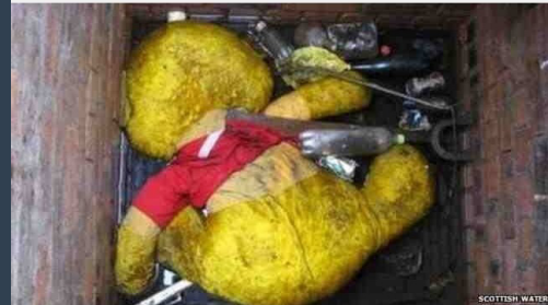
A Winnie the Pooh teddy bear was found dumped in a manhole in East Kilbride, South Lanarkshire
