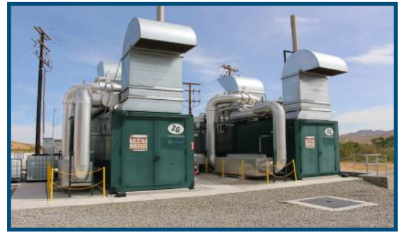
VWVRA uses two 800 kwh generators to convert biogas or methane into electricity.
