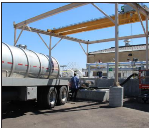
Activated sludge being delivered to the Hesperia Subregional for "seeding".
