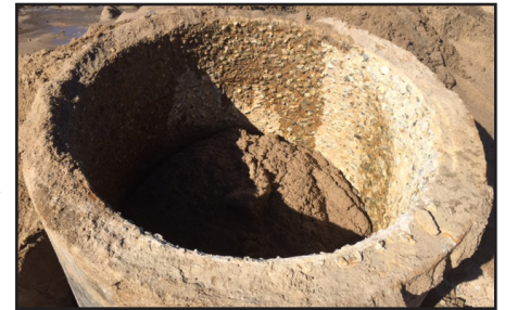
Old, damaged manhole.
