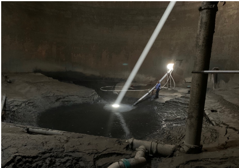
Inside a Regional Plant Digester
