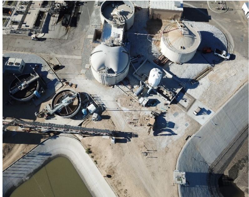
Regional Plant Digesters
