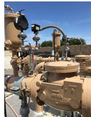
Hesperia Lift Station
