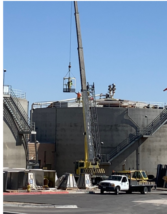
Regional Plant Digesters
