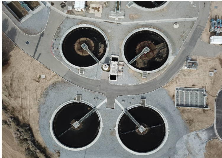
Regional Secondary Clarifiers
