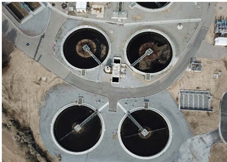
Regional Secondary Clarifiers
