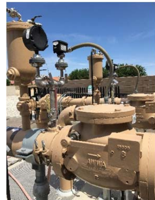
Hesperia Lift Station
