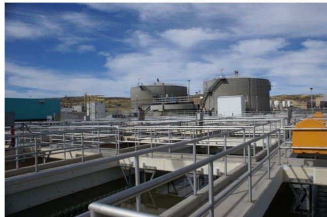
Regional Plant Digesters
