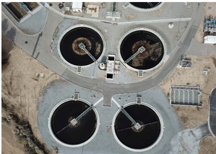
Regional Secondary Clarifiers
