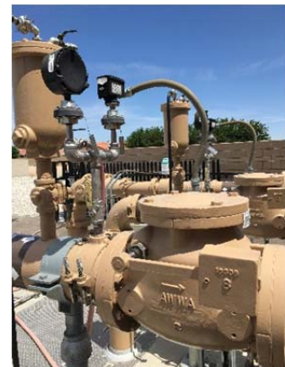
Hesperia Lift Station
