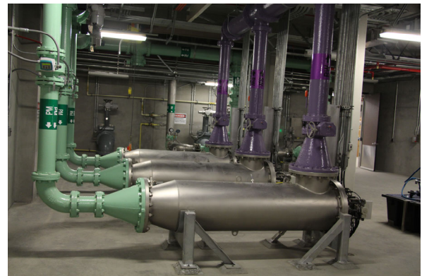
Equipment at the Hesperia Sub-regional Plant
