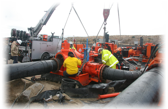
Coping with sewer overflow at Upper Narrows
