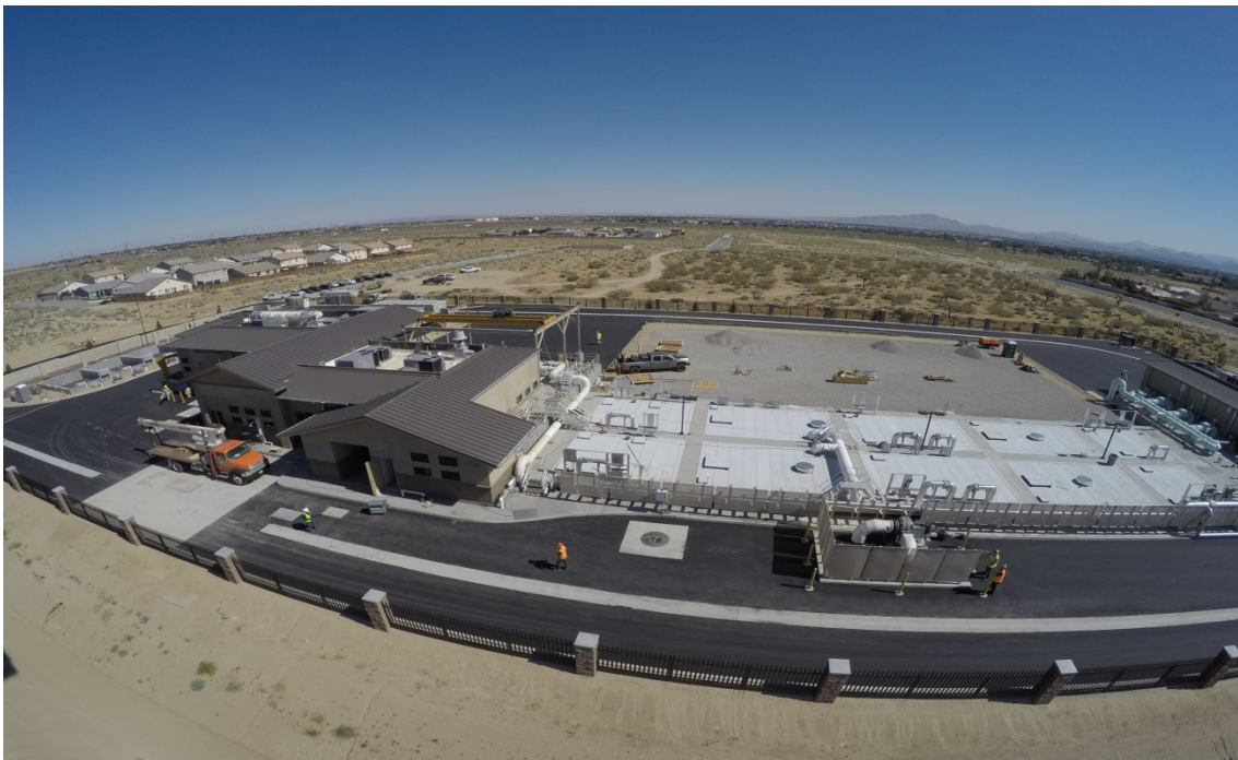
Hesperia Sub-regional Water Reclamation Plant
