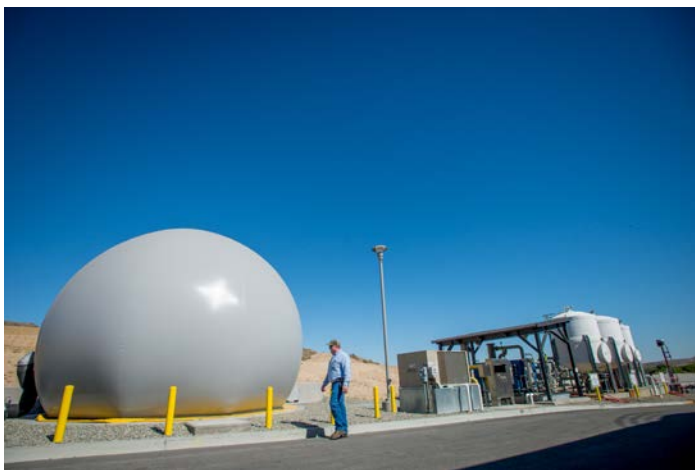
Biogas treatment and storage
