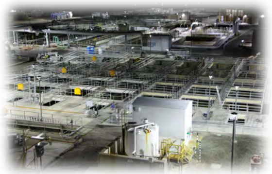
Wastewater Treatment Plant at night
