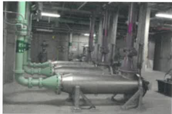
Equipment at the Hesperia Sub-regional Plant
