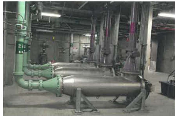
Equipment at the Hesperia Sub-regional Plant
