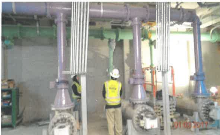
Hesperia Plant - the purple reclaimed water pipeline
