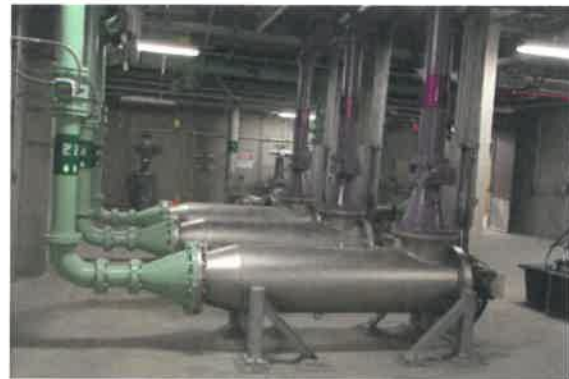
Equipment at the Hesperia Sub-regional Plant
