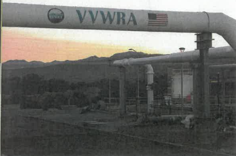
The Victor Valley Wastewater Reclamation Authority looks to become energy neutral by supplying its own energy needs onsite.
