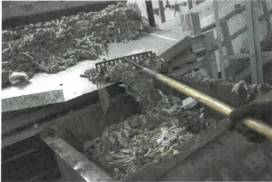
Raking wipers and other waste into a bin for disposal at the Newtown Creek Wastewater Treatment Plant in Brooklyn. Credit Credit Karsten Moran for The New York Times
