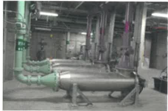
Equipment at the Hesperia Sub-regional Plant
