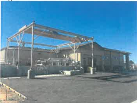
Apple Valley Wastewater Reclamation Plant
