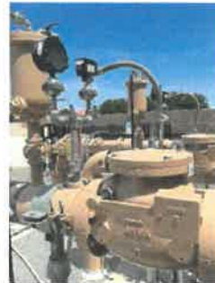
Hesperia Lift Station
