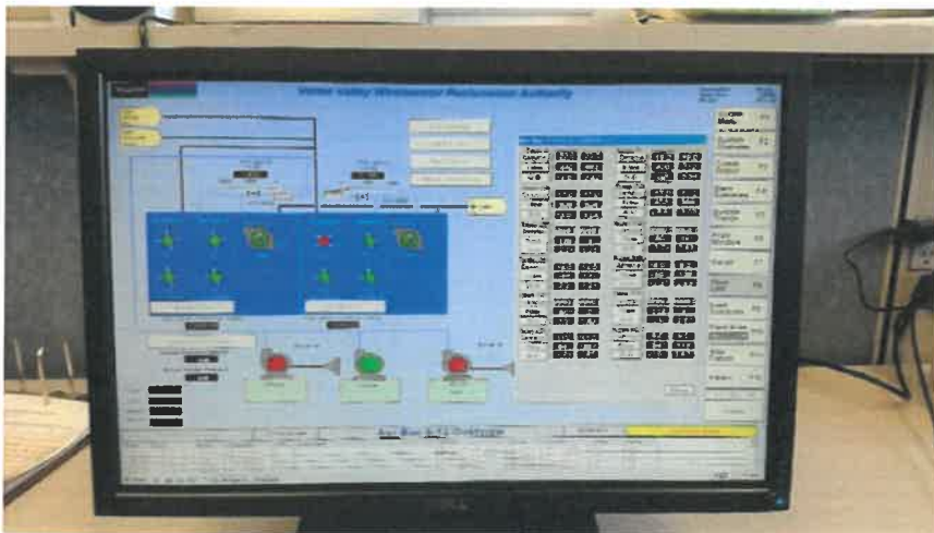
VWRA SCADA System
