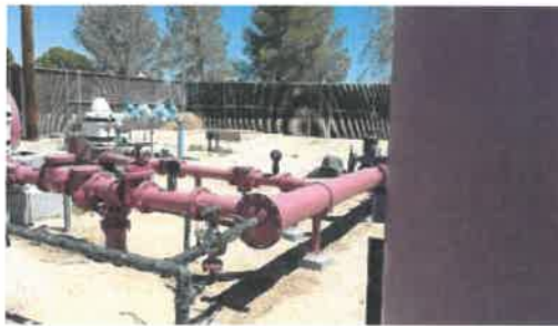
Recycled Water Pipelines
