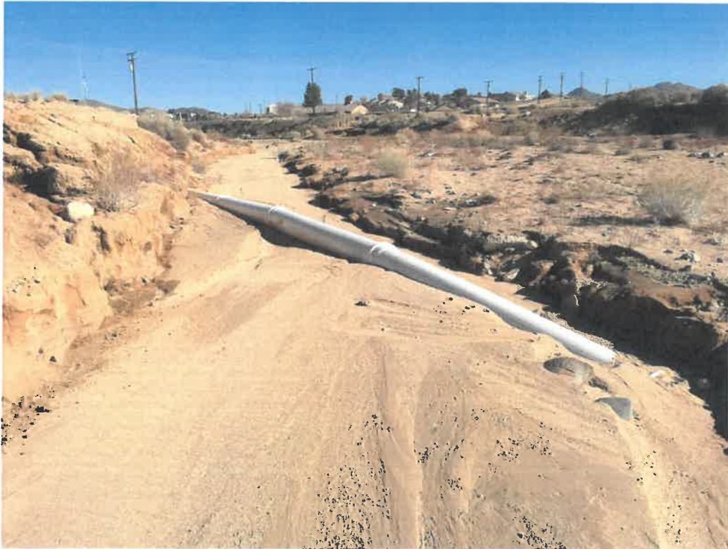
Desert Knolls Wash exposed due to the storm
