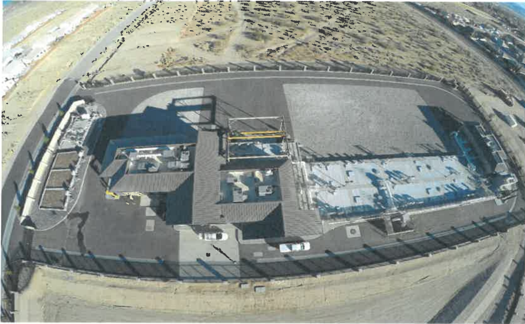
Hesperia Wastewater Reclamation Plant
