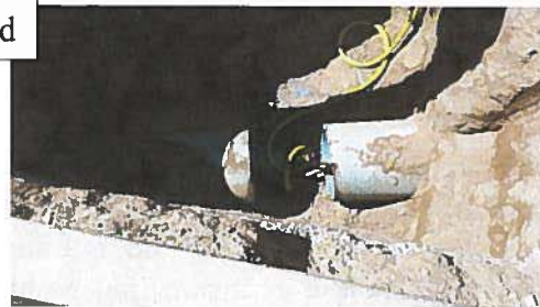
Figure 4 Storm Drained Cut and Plugged. This will be Blind Flanged.
