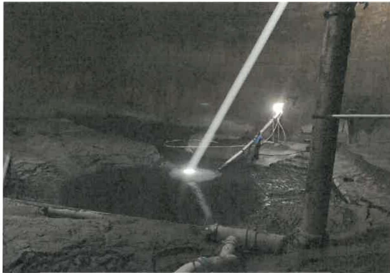
Inside a Regional Plant Digester
