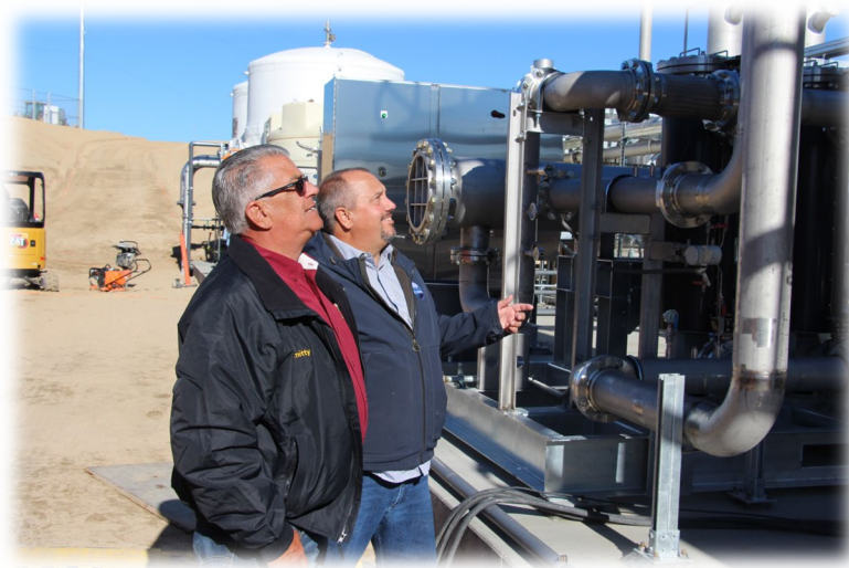
Renewable Gas Project at Victorville Plant
